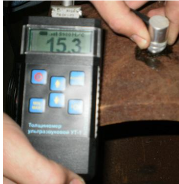
Measure the wall thickness of the corroded surface
